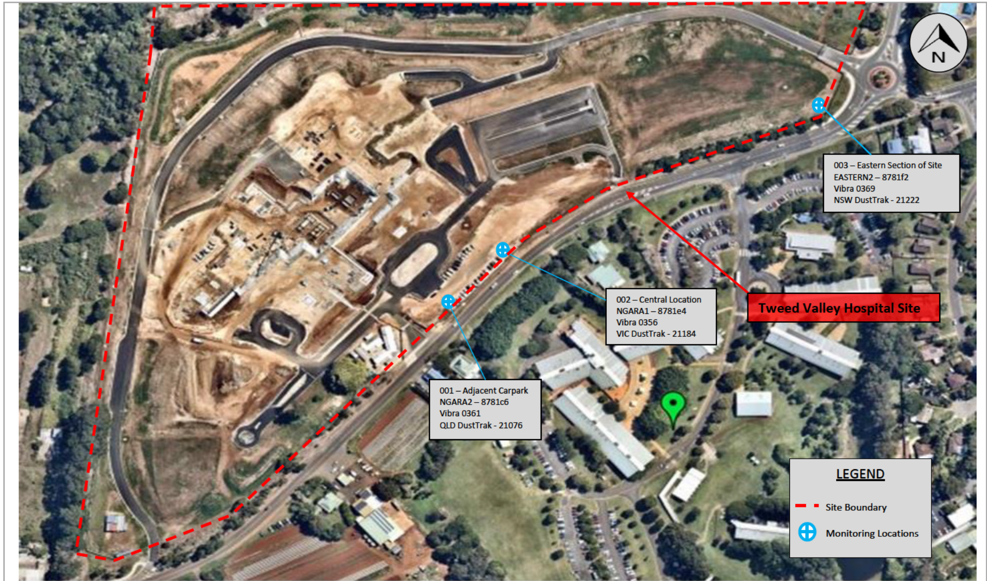
Aerial photograph of the Tweed Valley Hospital Project at Cudgen, NSW (as of 30 November 2020).
