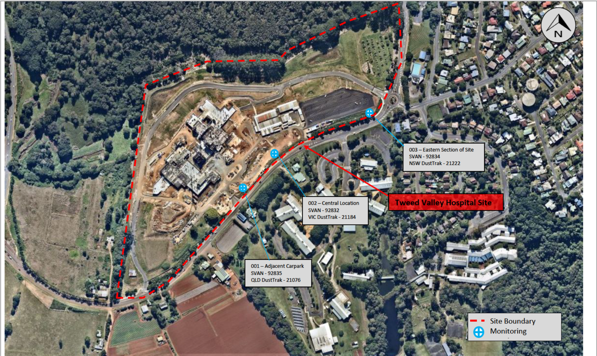
Aerial photograph of the Tweed Valley Hospital Project at Cudgen, NSW (as of 6 th of June 2021).
